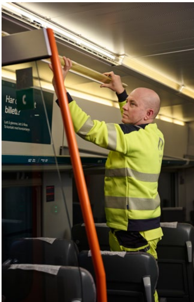
Hans Ingar Fossen dismantling an old light tube containing mercury. They are to be replaced with new led lights.
